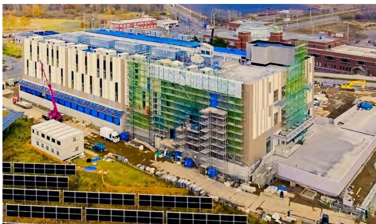
Ishikari Renewable Energy Data Center 1; Construction photo taken in November Courtesy of Ishikari Renewable Energy Data Center LLC No. 1
